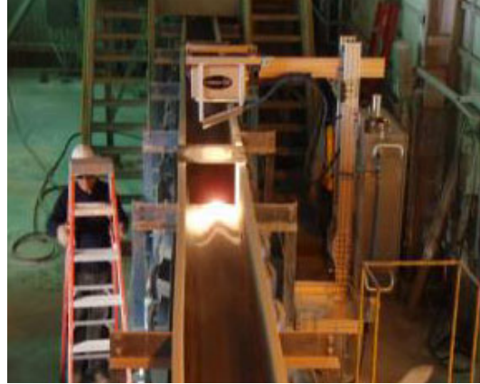
Figure 12. Lime mud solids analyser installation on a mud-feed line feeding a kiln. The probe-head is mounted 29" above the sample surface with an illumination spot of 6".
